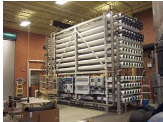
City of Bowling Green Water Treatment Plant
