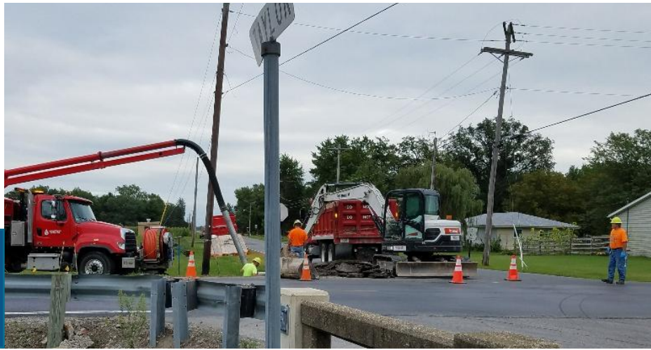
District crews repair a water leak in Weston. The District continues to correct issues with aged water lines in the area, while replacing problem lines with construction projects. More work will take place over the next few years to upgrade this system.
