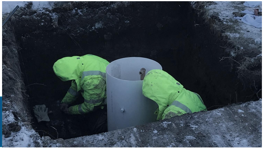
Above: Crews dig a new meter pit in Portage following a water line break during recent arctic weather. With safety a priority, crews take warming breaks to reduce exposure to the cold.
